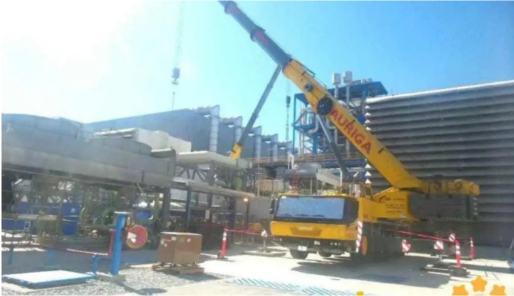
Olague electromechanics turbine support sa de cv delicias
